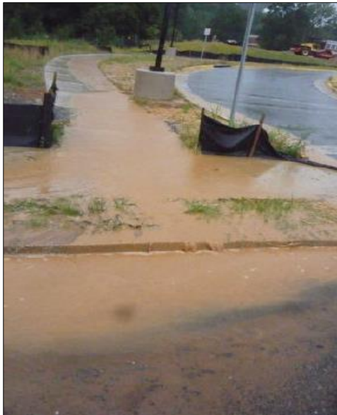
7/27/15 flooding, erosion and runoff on the Ashlawn site
