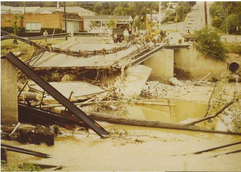
Walter Reed bridge destroyed by flooding in 1972
