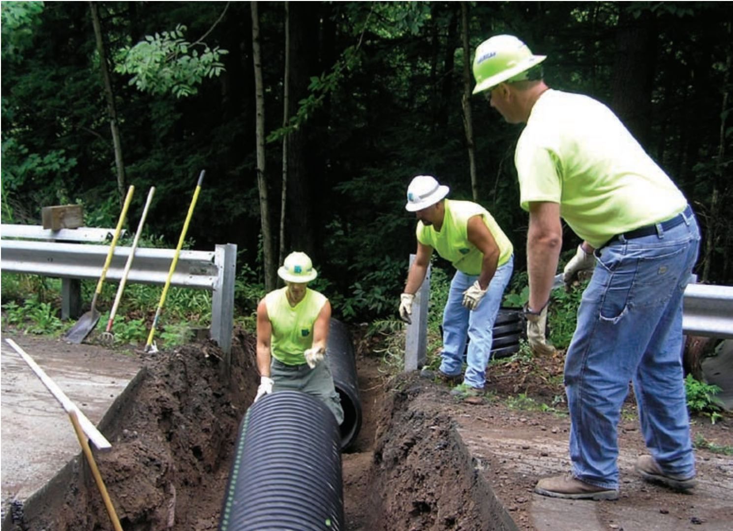
PennDOT workers lay replacement drainage pipe as part of a road maintenance project. Proper drainage for streams that cross beneath roads is a critical maintenance step.
