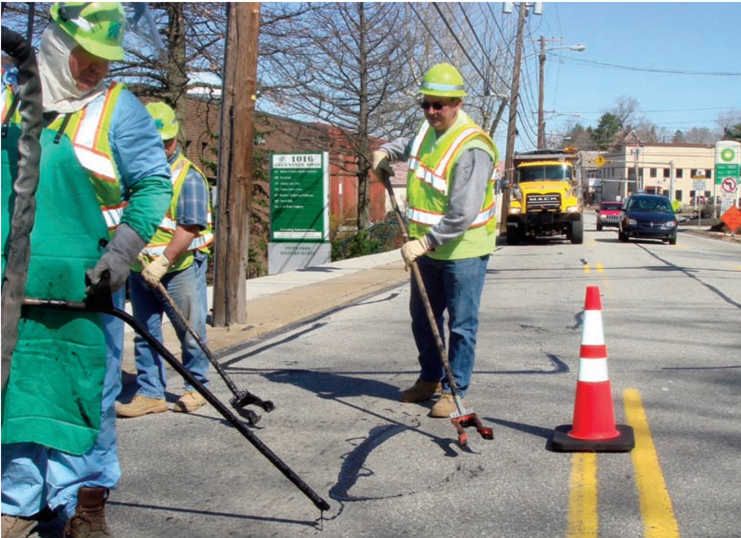
PennDOT workers engage in crack sealing to keep moisture from penetrating beneath the road surface. In Pennsylvania, which has a vigorous freeze-thaw cycle each winter, keeping moisture out of the area beneath road surfaces is a critical maintenance step.
