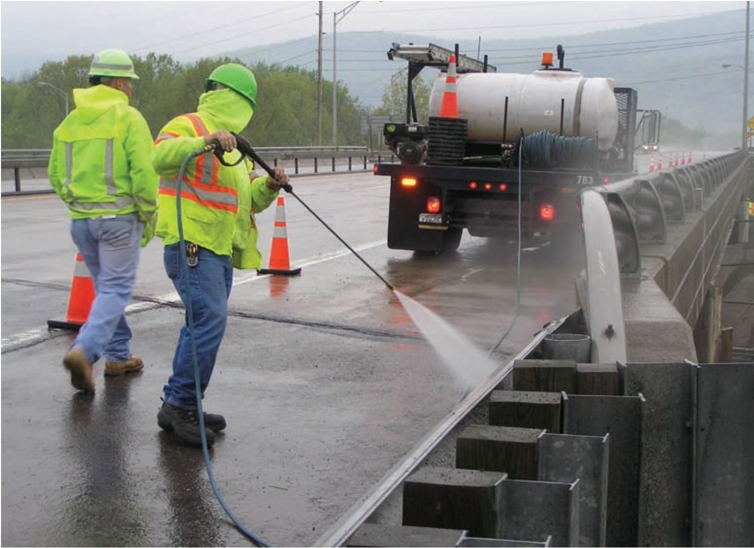
PennDOT workers power wash a bridge structure. Keeping the expansion areas and joints of bridges free of debris and salt accumulation from winter services is a critical maintenance function.
